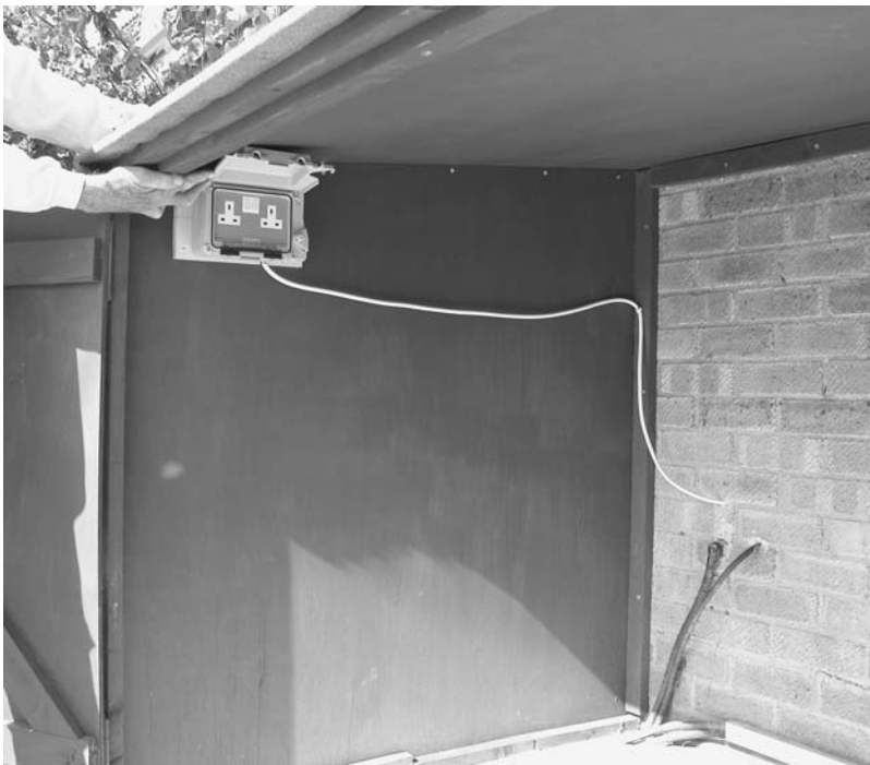
Figure 9.11. Electrical supply in the shelter.
