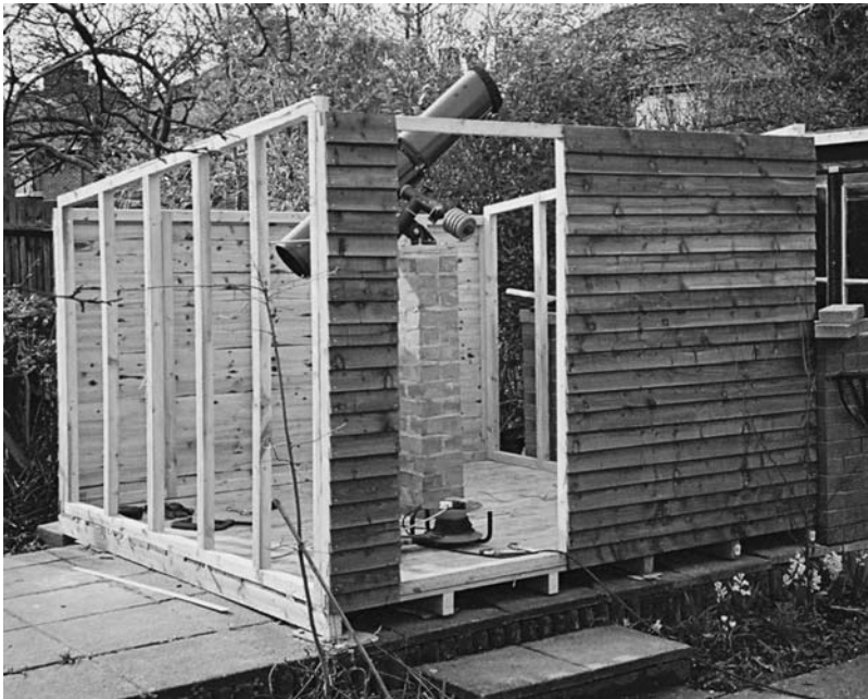
Figure 9.22. Shed partially assembled, showing unclad wall-frames, and 6.25 in. telescope experimentally in place on the first, unsuccessful, pier.
