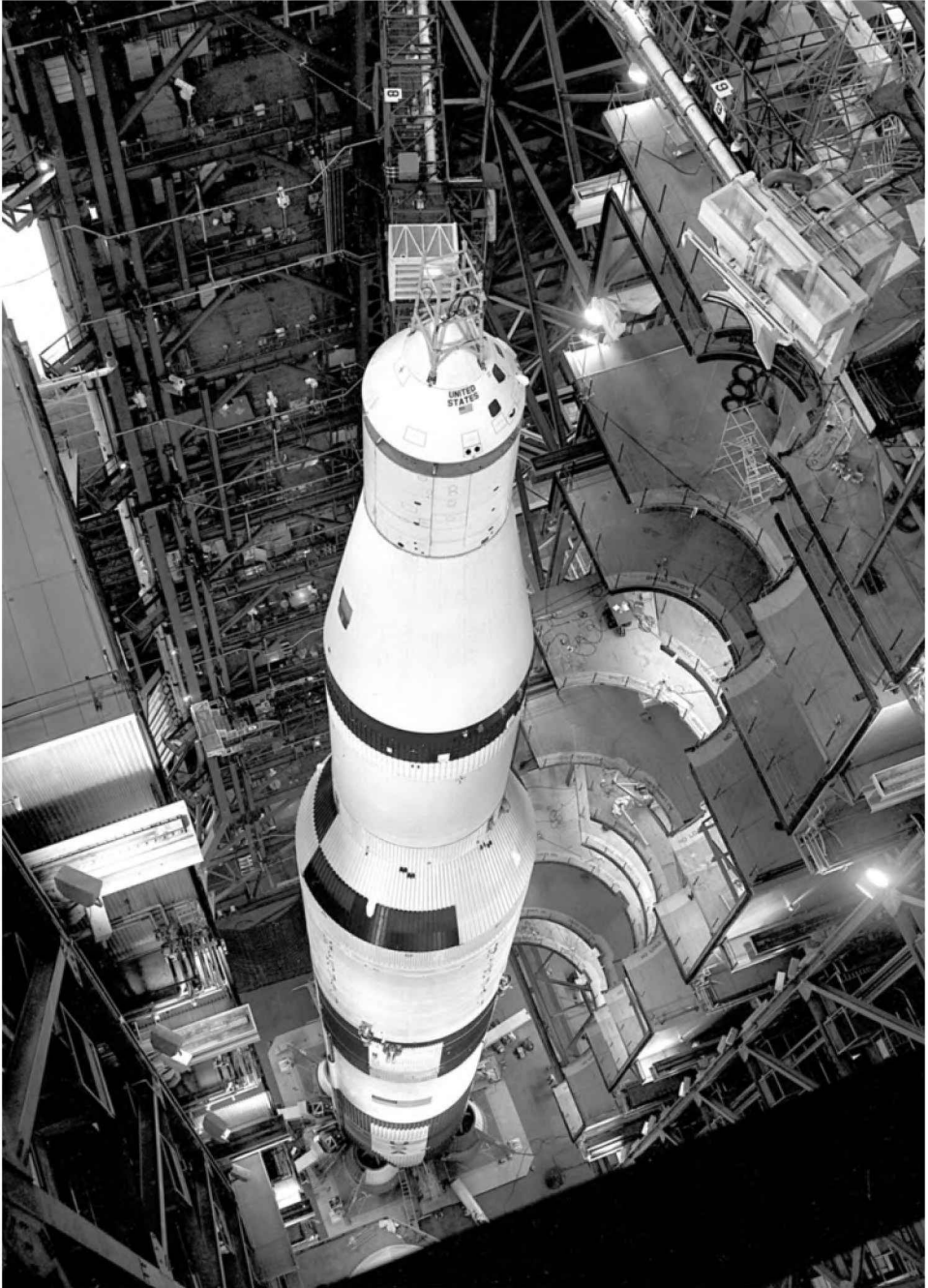
AS-501, the first flight of the Saturn V, topped by the Apollo 4 command and service module, is prepared in the VAB for its November 1967 launch.
