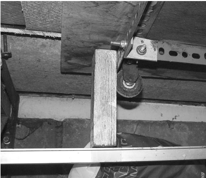
Figure 9.2. The rail and block arrangement holding up one corner of Bob's rolling roof, in the closed position.
