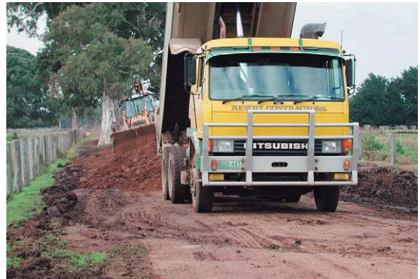
Figure 8-6 Tracks should be properly constructed. The first step is to create a base of well-compacted, crushed rock fill. The finished track surface should be above that of the surrounding ground. (Courtesy of J Malmo)
