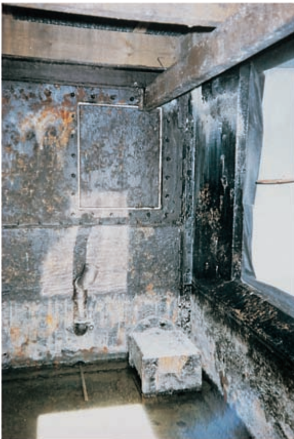
Figure 25.5 Inside view of a cooling tower – a potential source for Legionella pneumophila . This badly maintained tower was the source of a large outbreak of legionnaires' disease.
