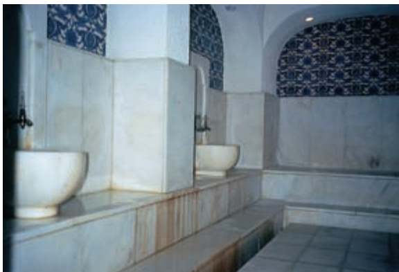
Figure 7.9 Poorly maintained Turkish bath in a hotel that caused an international outbreak of legionnaires' disease: 11 people from four countries contracted the infection.
