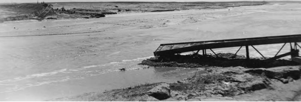
Railroad bridge destroyed by a 1935 flood on the South Platte River in Fort Morgan, Colorado, twenty-five miles south of the Pawnee National Grassland. Note the wide, shallow channel and the complete absence of trees and shrubs along the stream banks. Courtesy, Colorado Historical Society.
