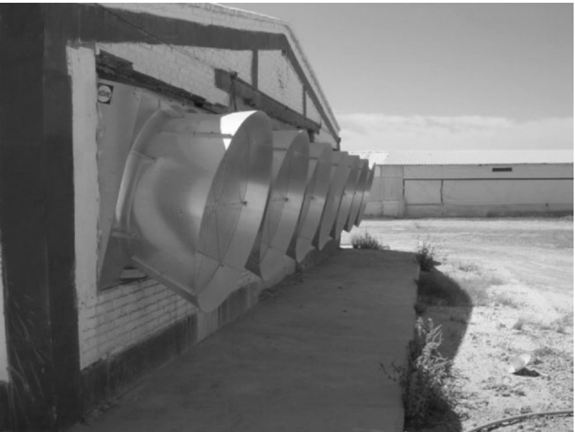
Fig. 5.31. Discharge cone fans.
