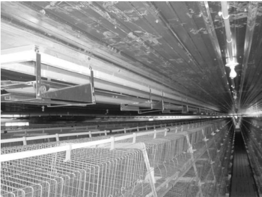
Fig. 5.19. Slot attic inlet in commercial layer house.
