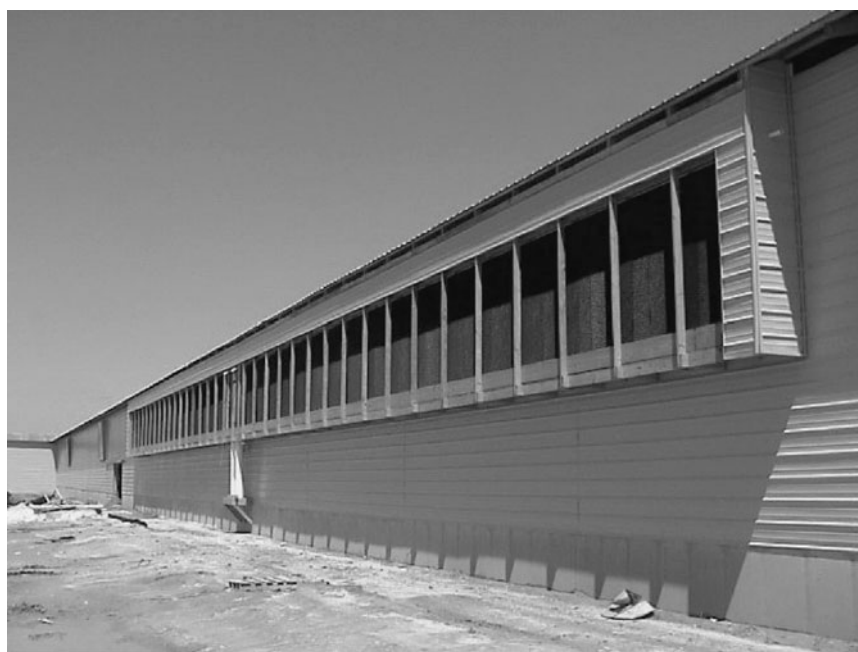
Bi-directional tunnel-ventilated house with evaporative cooling pads in the centre.
