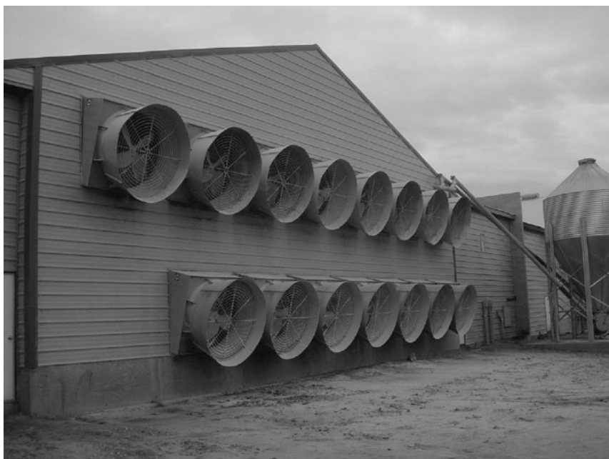
Bi-directional tunnel-ventilated house with fans.
