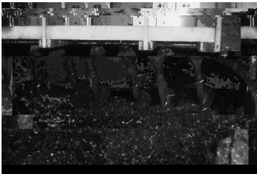
Fig. 2.6. Augers mixing a full digester (Delaware, USA).
