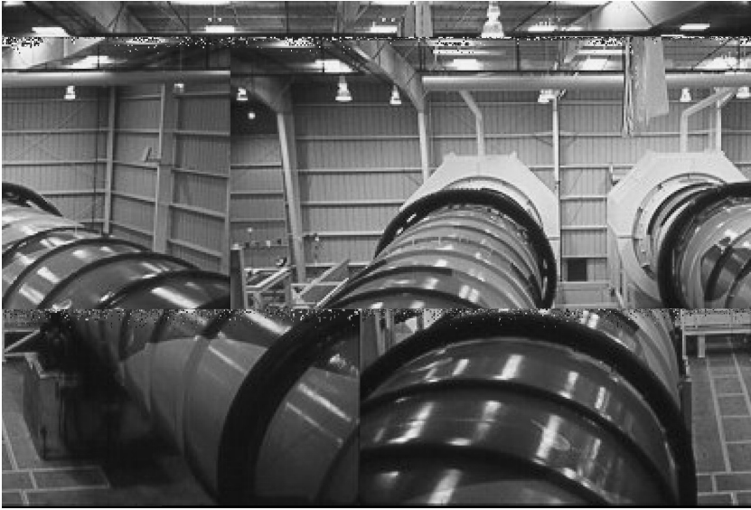
Fig. 5.8. View of a typical rotating drum.
