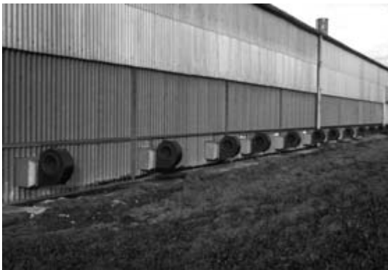
Fig. 3.12 External view of a floor store showing a row of aeration fans used for cooling, each fan serves one under-floor duct (UK) (see Fig. 3.11).
