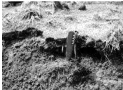
Photo 6. Soil erosion and ceiling caused
