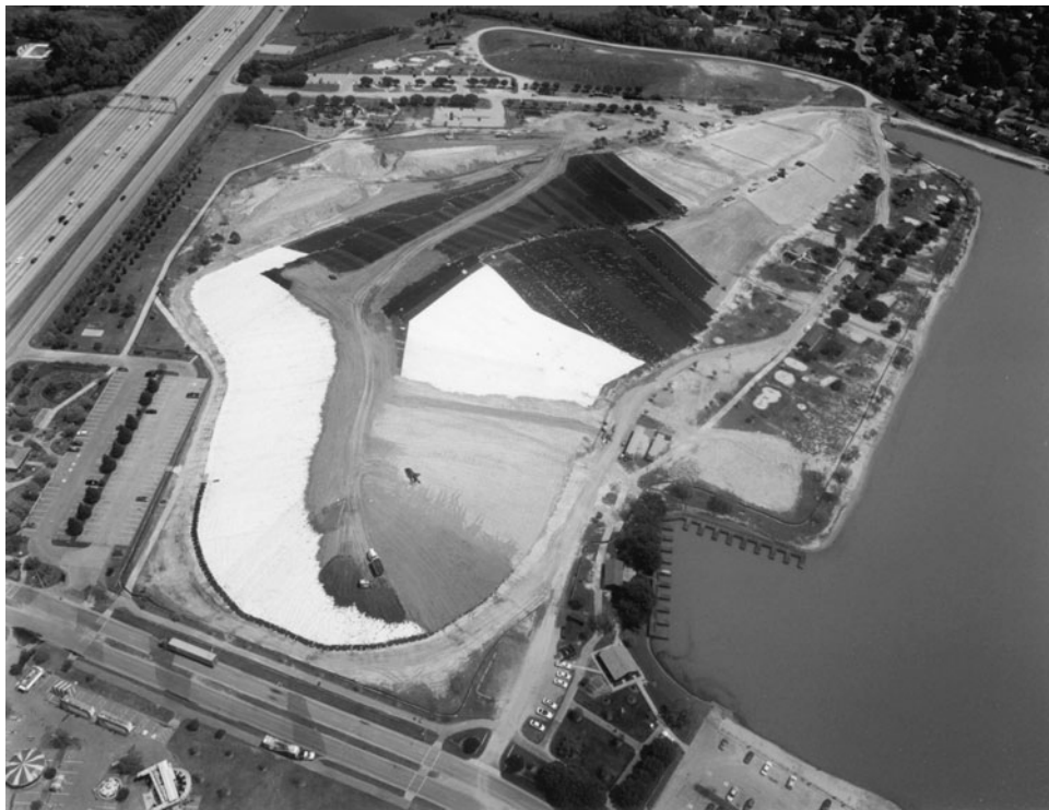
FIGURE 5.10 Aerial view of the proper closure of a modern-day landfill, which is required by strict environmental regulations. The landfill is being covered by several layers of materials to prevent rainfall infiltration and leaching, and to ensure no future adversarial impact on groundwater resources. Note the highway on the left for scale. (Printed with permission of the City of Virginia Beach, VA, the United States.)
