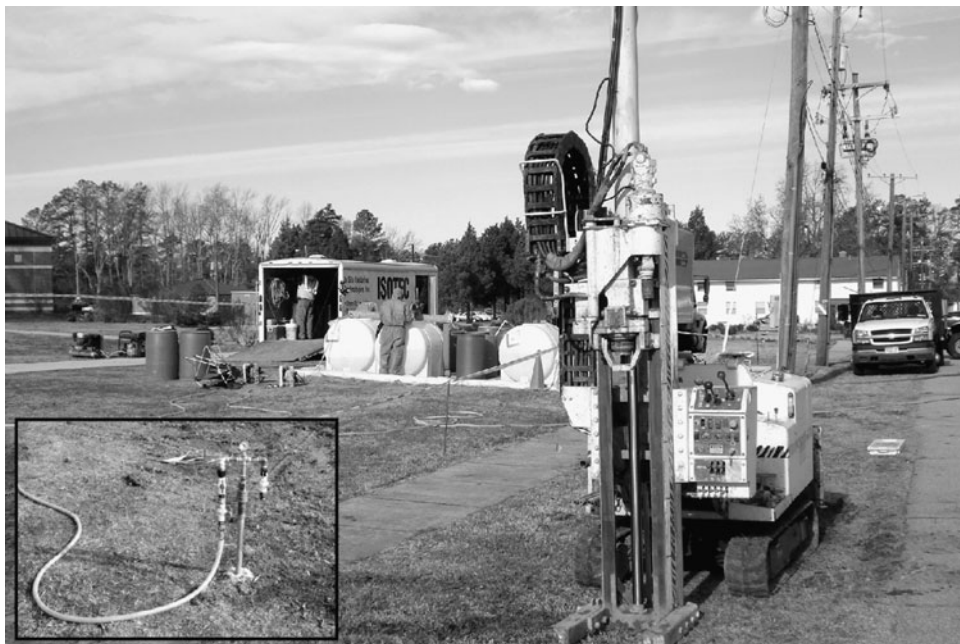
FIGURE 9.32 Direct-push drilling for oxidant injection into shallow aquifer contaminated with chlorinated solvents. Inset: Temporary injection point with the oxidant feed line. (Photographs courtesy of ECC)
