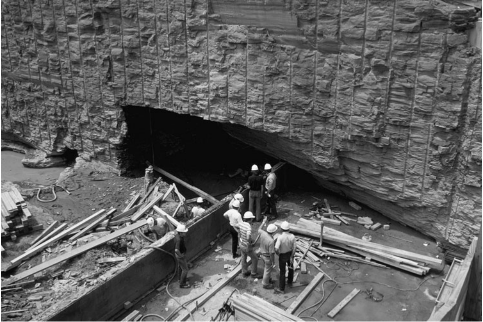
FIGURE 2.83 Large cavity at a construction site in Paleozoic limestone, Hartsville, TN. The matrix porosity is measured at 2 percent. (Photograph by George Sowers; printed with kind permission of Francis Sowers.)
