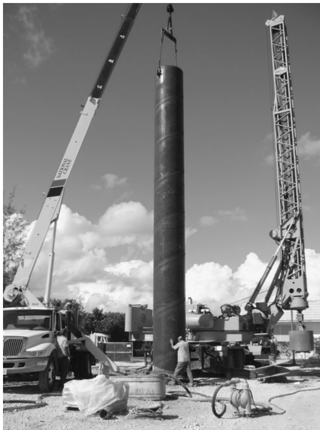
FIGURE 7.3 A 48-in.-diameter surface casing being placed in a 54-in.-diameter borehole. The target depth for the well is 1300 ft with an open interval from 1000 to 1300 ft in the Floridan aquifer. The final casing inside diameter is 20 in. The well is drilled for water supply of the city of Miramar, FL. (Photograph courtesy of Richard Crowles.)
