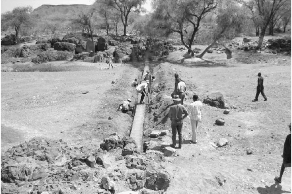
FIGURE 7.23 Construction of subsurface dam in Turkana District, Kenya, constructed by compacting clay in the narrow trench (dyke). (Photograph courtesy of VSF-Belgium, 2006.)
