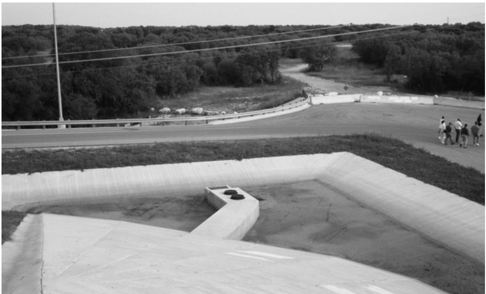
FIGURE 8.25 Concrete catch basin by a state highway in Austin, TX, designed to strip oil and fines from surface runoff before water is allowed to infiltrate into the underlying Edwards aquifer.
