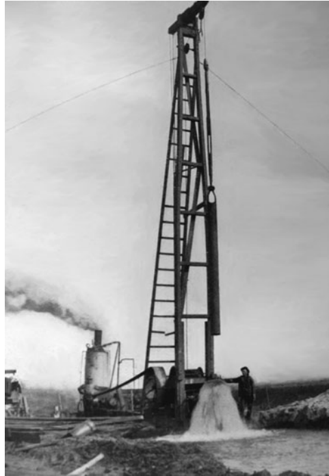
FIGURE 7.2 California well rig after completing 12-in. well flowing 5,250,000 gallons per 24 hours. (From Slichter, 1905; photograph courtesy of U.S. Geological Survey.)
