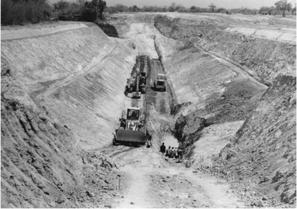
FIGURE 7.28 Construction of one of the largest subsurface earth-fill dams in Africa located in Nare Village, Burkina Faso. (From Ministry of the Environment, 2004.)
