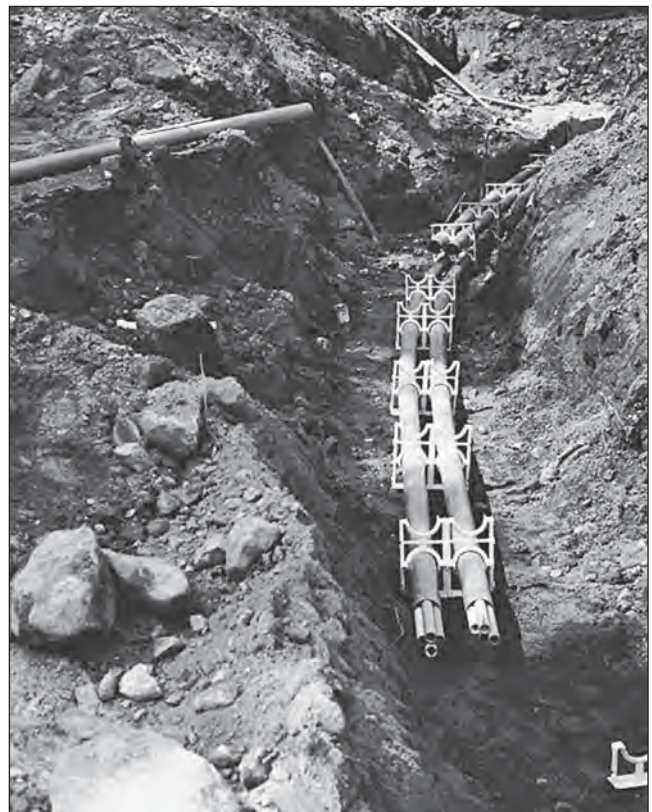
FIGURE 26.12 Inner duct photo.
