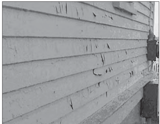
FIGURE 17.2 Lead-based paint peeling from a structure.
