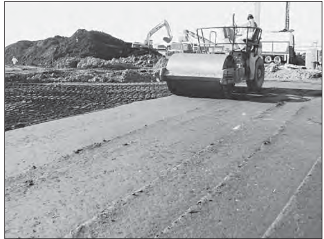
FIGURE 17.9 Placement and compaction of stabilized soil as pavement subgrade. (Reprinted with permission of Pollution Engineering © 2002)
