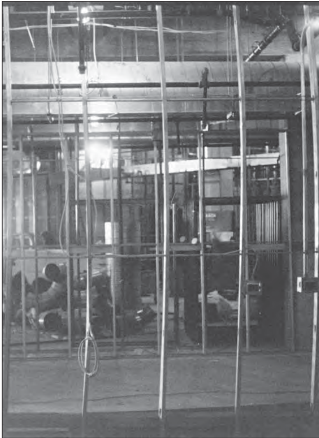
FIGURE C.16 Photo of frost heave damage to a concrete floor slab.
