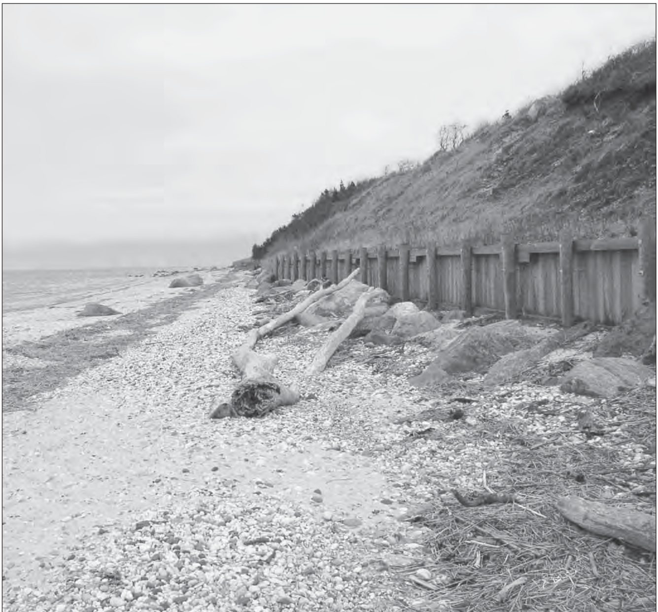
FIGURE 27.14 Wooden bulkhead for bluff recession stabilization. (Photo courtesy of Brian K. Batten, PhD)
