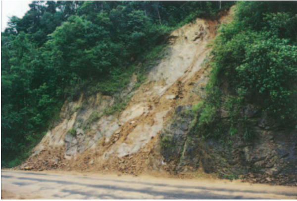
Figure 32 Landslip erosion on steep slope. (Photo: Michelle Batko)
