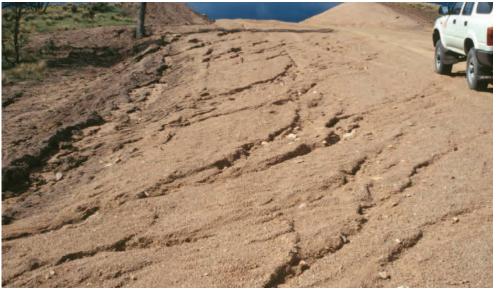
Figure 28 Rill erosion. (Top) Soil is deposited in the delta from rill erosion (Photo: Bruce Carey). (Bottom) Rill erosion on the roadside (Photo: Michelle Batko).
