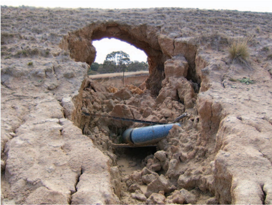
Figure 30 Tunnel erosion in a pasture (top) and through a dam bank (bottom). (Photo: Michelle Batko)
