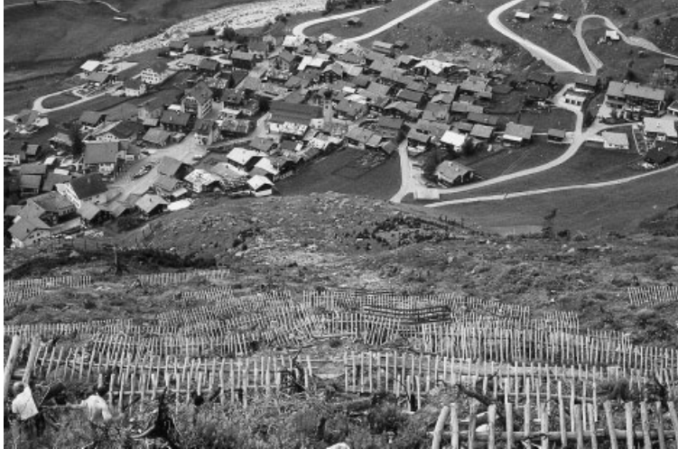
Fig. 3.3 Temporary avalanche barriers established after storm damage, protecting the village of Curaglia, central Switzerland.
