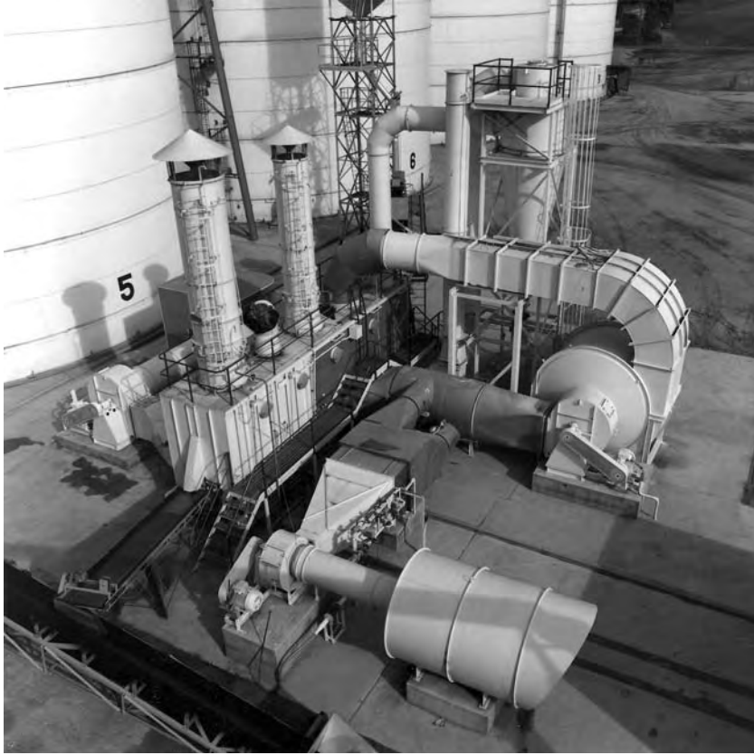
Fig. 8.9. Continuous-flow fluid bed heat disinfestation plant (150 t/h capacity) in Victoria, Australia.
