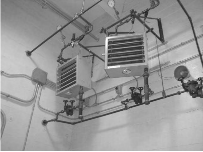
Fig. 8.14a. Fixed steam heater used in food-processing facilities.
