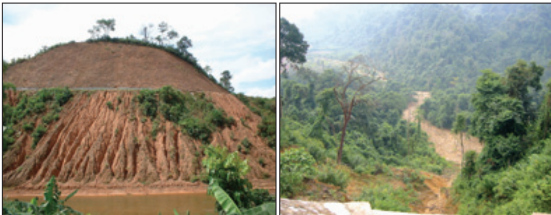
Photo 20: Left; If not properly protected rock/soil from this waste dump will wash far downstream. Right: impacting a downstream village in A Luoi district, Thua Tien Hue province.
