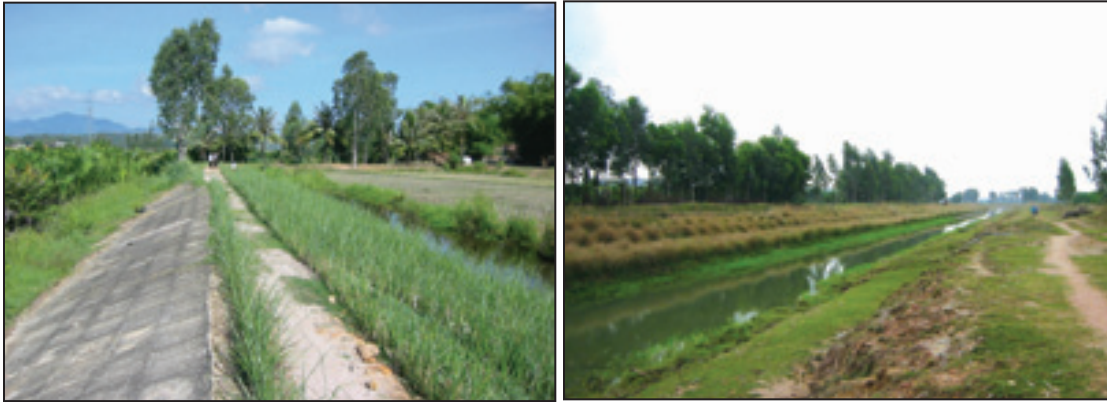
Photo 12: Upstream anti-salinity dike section with traditional concrete riprap facing the river (left) and along a section of the irrigation canal, surface erosion mars the opposite bank (right).
