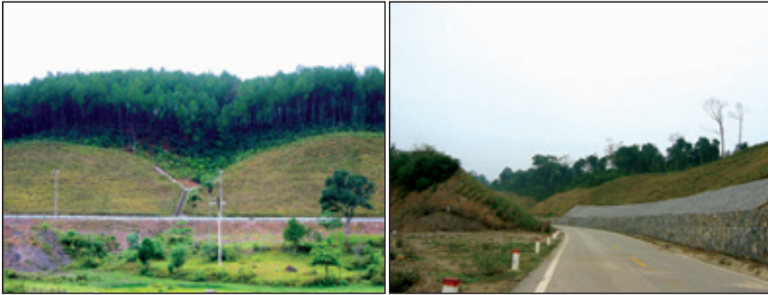
Photo 19: Left: Vetiver stabilizes cut slopes along the Ho Chi Minh Highway; right: both alone and in combination with traditional measures.
