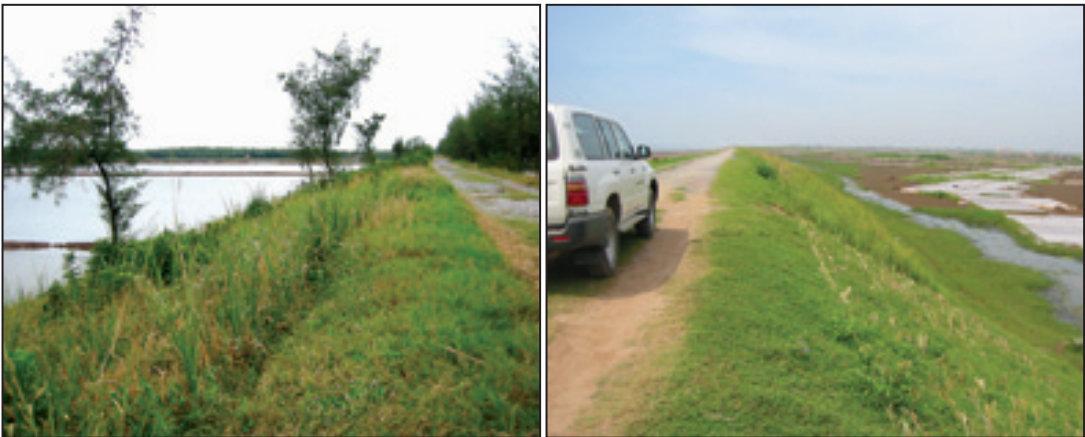
Photo 18: In North Vietnam; left: Vetiver planted on outer side of a newly built sea dike in Nam Dinh province; right: on the inner side of the dike, planted by the local Dike Department.
