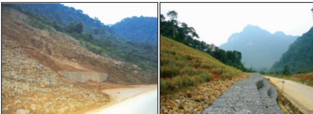
Photo 21: Da Deo Pass, Quang Binh: Left: Vegetation cover is destroyed, revealing ugly and continuous failures of cut slopes; right: Vetiver rows on top of the slope very slowly squeeze down, considerably reducing the failed mass.
