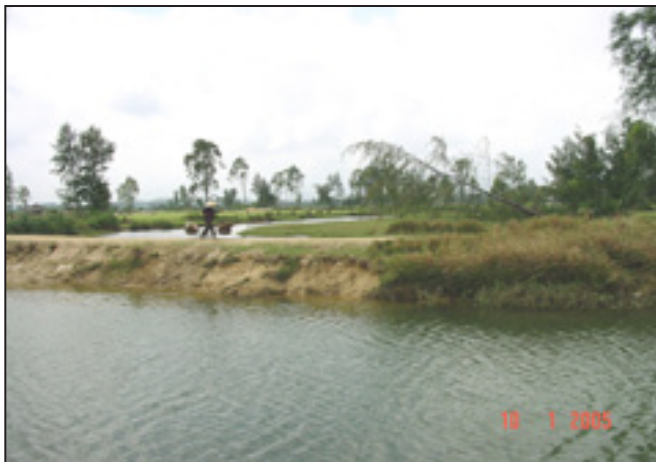
Photo 23: The right section of this rural road in Quang Ngai is protected by vetiver; the left section is unprotected.
