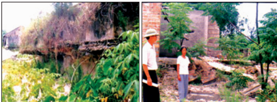
Photo 2: Sand flow in Le Thuy (Quang Binh) in 1999: the foundation of a pumping station (left) and the foundation of this woman’s three-room house is being undercut by moving sand (right).
