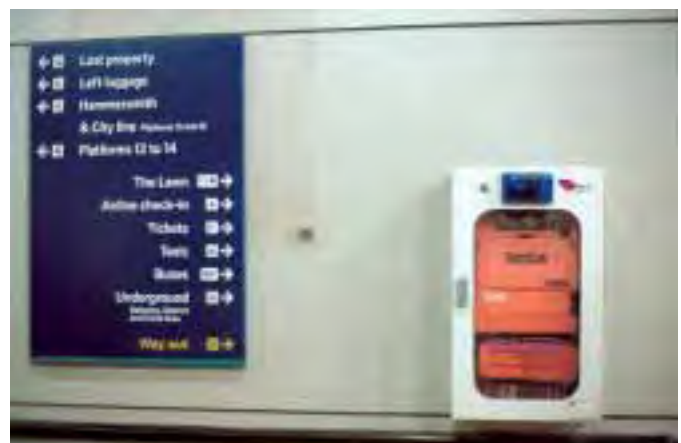
AED on a railway station
