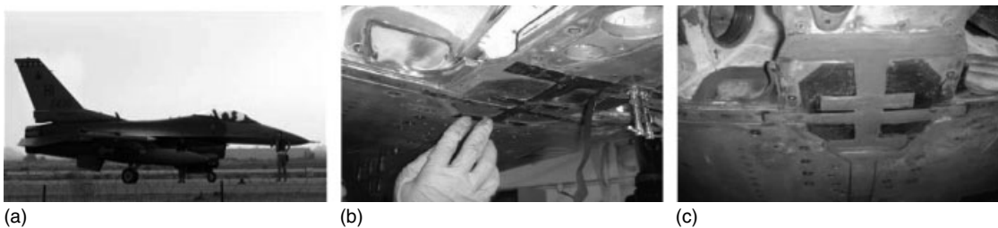
Figure 10. The SMART Layers were mounted on the three repairs installed in the keel area of the station 341 bulkhead. (a) In-service F-16, (b) installation, and (c) mounted SMART Layer with surface coating [21].
