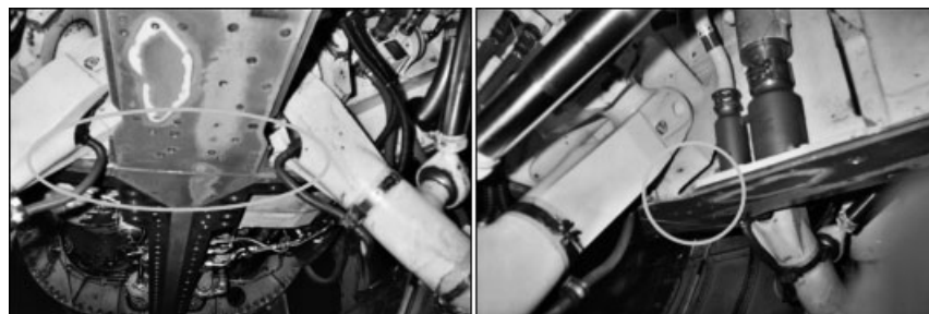
Figure 1. The main landing gear wheel well of an F-16 contains complex structure and multiple system installations.
