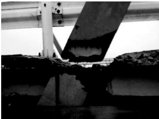
Figure 13. Kisogawa Bridge defect.
