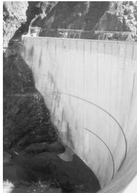
Figure 34. Photo of Mauvoisin dam downstream face. The “air ladders” mentioned in Section 4.5 can be seen.
