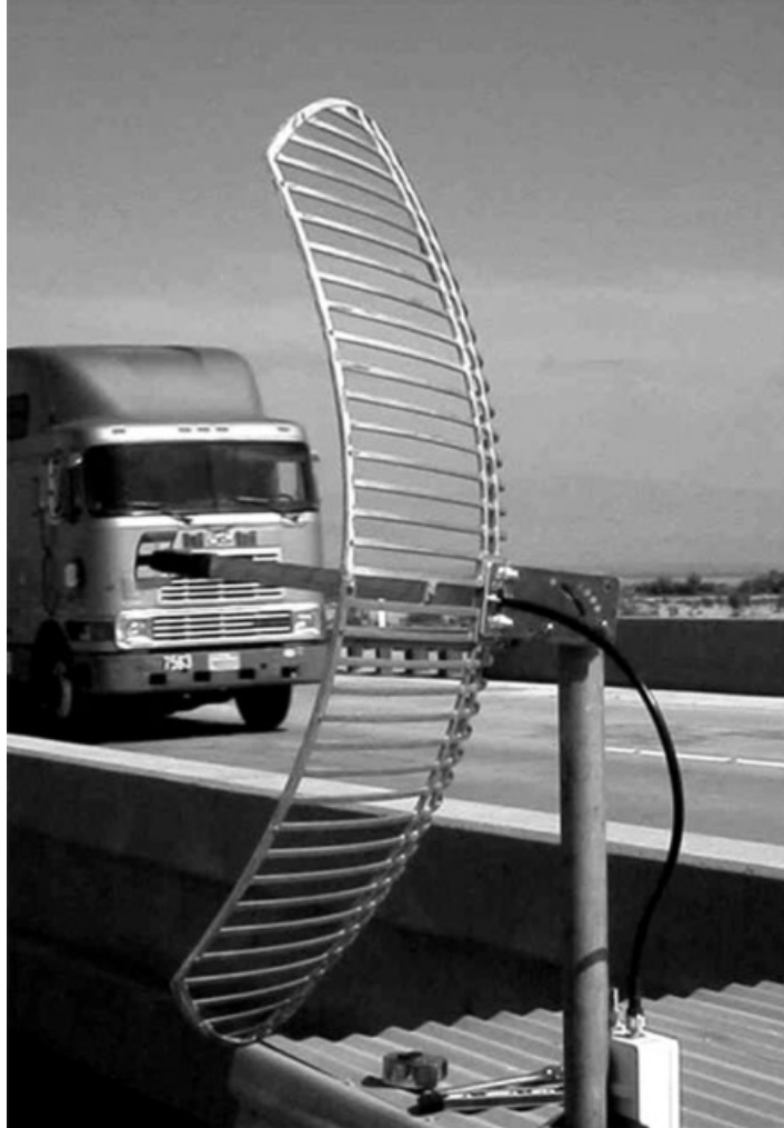
Figure 6. Bridge with antenna for data transmission.
