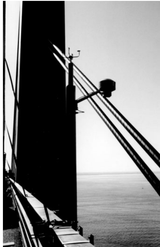
Figure 7. Weather station at the deck level of the bridge.
