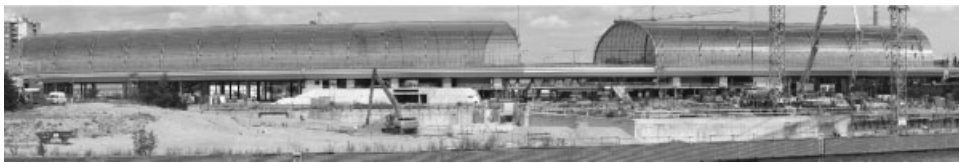
Figure 2. New modern main station Lehrter Bahnhof with flat glass arch roofs during construction in 2003.
