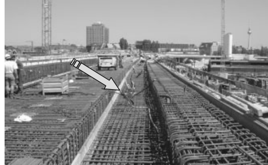
Figure 3. The cable tubes for the sensors were fixed in the structure before the concrete (see arrow).
