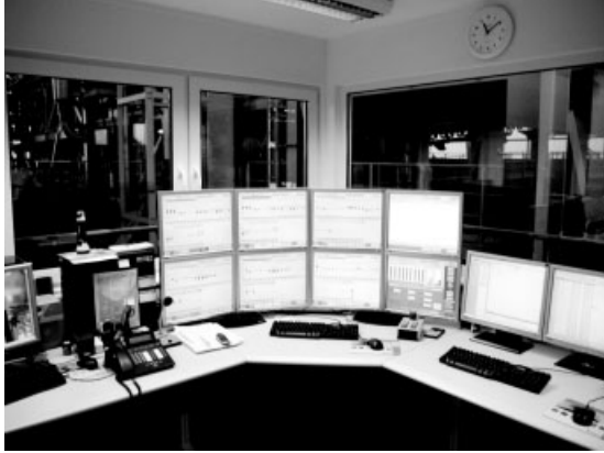
Figure 9. Operator view of the A380 EF control and monitoring system.
