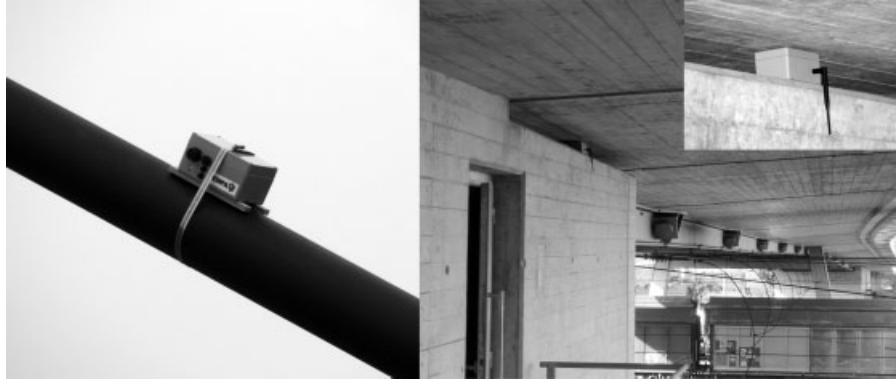
Figure 5. Views of a sensor node mounted on a cable and the root node in the bridge abutment below the bridge deck.
