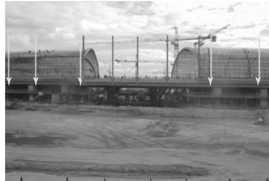
Figure 5. View of the monitored bridge of the main station during the construction phase. dark: laser displacement sensors; white: hydrostatic leveling system.
