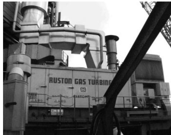
Figure 6. GTE enclosure on a rig.
