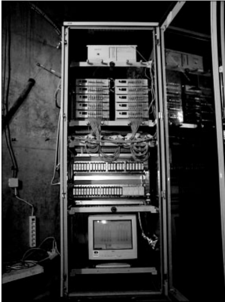
Figure 12. System centralization cabinet.
