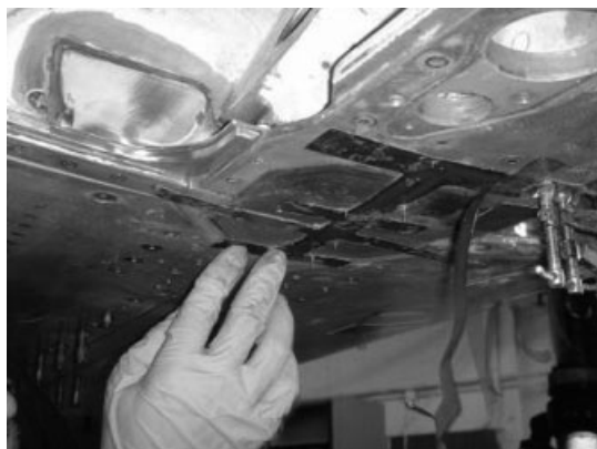
Figure 3. The sensor was carefully wrapped around the repairs, positioned, and adhered to the structure.
