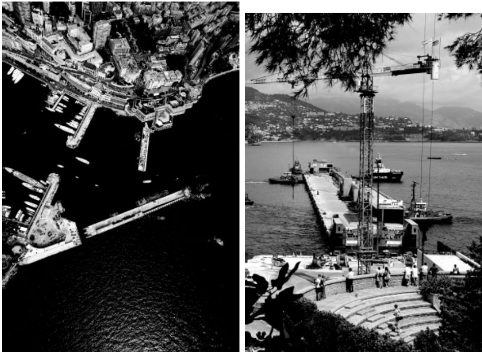
Figure 18. Views of the approach process for the final installation of the dock in Monaco.
