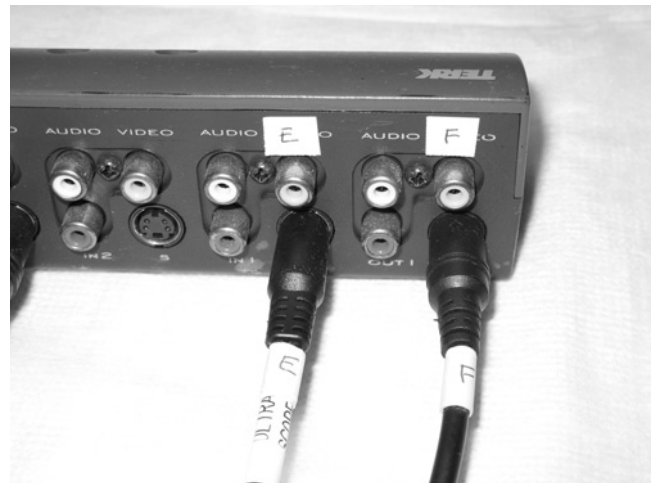
Figure 3.6 Keeping both wires and their receptacles clearly labeled helps ensure quick and accurate hook-ups after equipment is moved for room cleaning.
