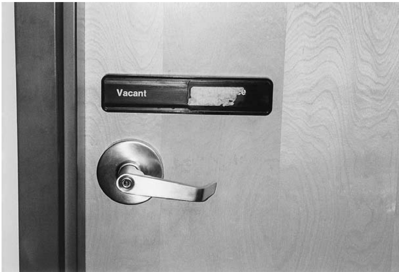
Figure 8.4. Bathroom Door with Vacancy Sign.
