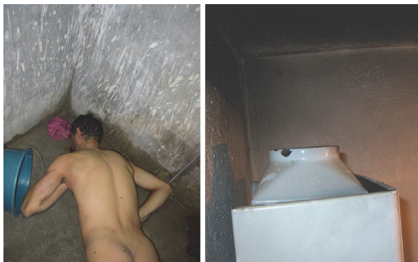
Fig. 24. A 42-year-old man was found dead due to carbon monoxide poisoning in his bathroom. There was an LPG water heater which had not a smoke pipe in the bathroom.
