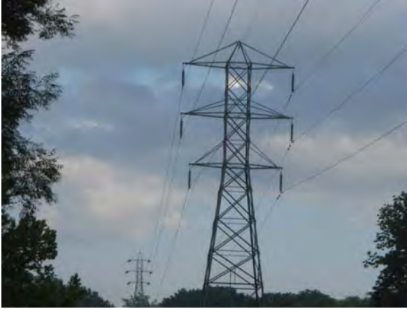
Fig. 17.3 High-tension power lines (greater than 100,000 V)
