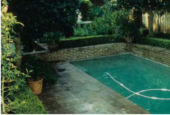
Fig. 16.15 A scene photograph showing a swimming pool in which a combined drowning/electrocution death occurred. The electric wiring of the pool lights was corroded such that the water was electrified
