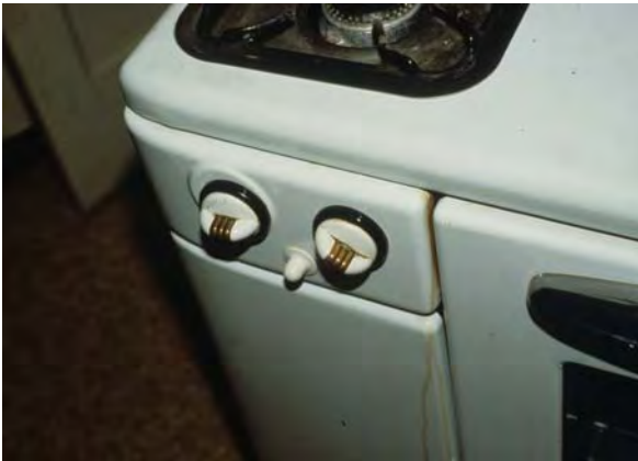
Fig. 11.31 An elderly woman was found dead in her home, which was filled with natural gas. A stove burner was in the “on” position, but the pilot light was extinguished
