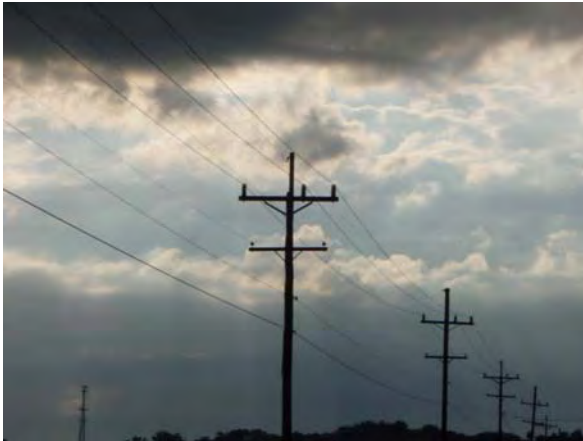
Fig. 17.2 Residential power lines (around 7500 V). Note that, in most instances, these power lines are not insulated (they are not coated with rubber)
