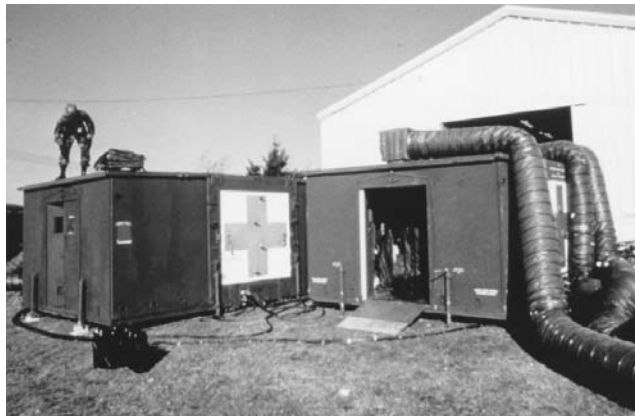
Figure 9-9 External view of air-transportable self-contained field x-ray facilities expanded and in use with generator cables and air-conditioning hoses.
