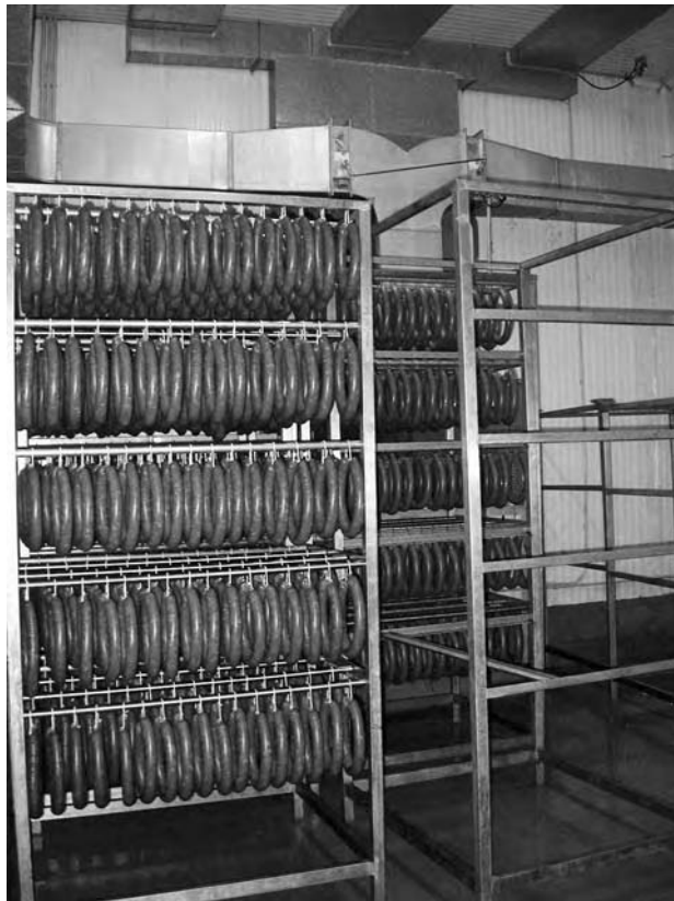
FIGURE 181.4 Example of a fermentation chamber with computer control of temperature, relative humidity and air rate. Courtesy of Tabanera Company, Segovia, Spain.
