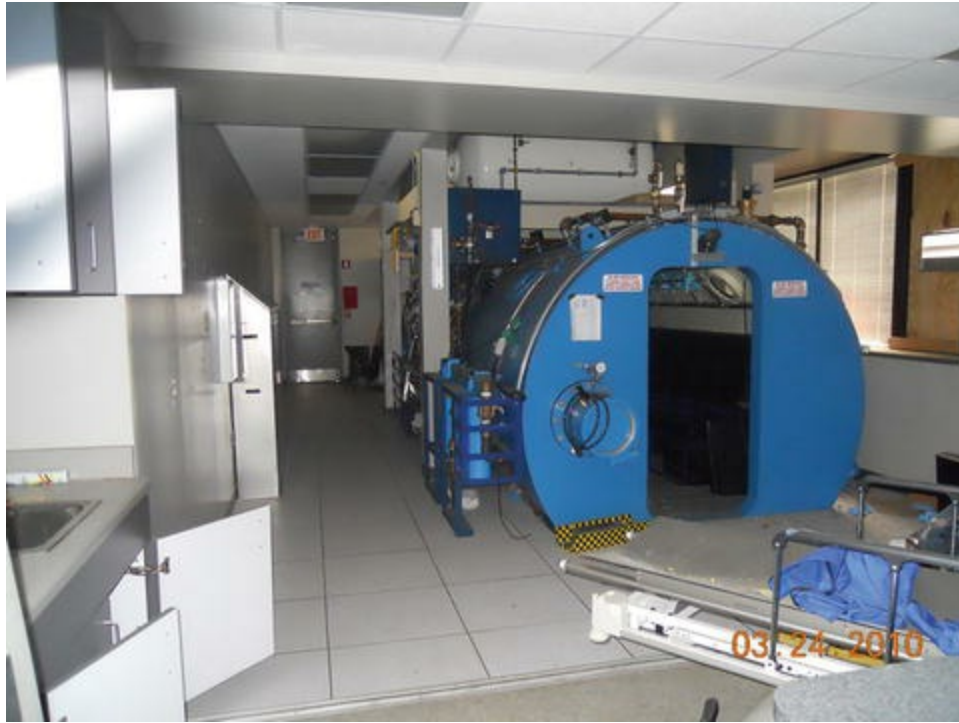
Fig. 42.20 Shown is a multiplace hyperbaric chamber with SICU/ICU capability in the Emergency Department at Charity Hospital's Trauma Center in 2005 in New Orleans, Louisiana
