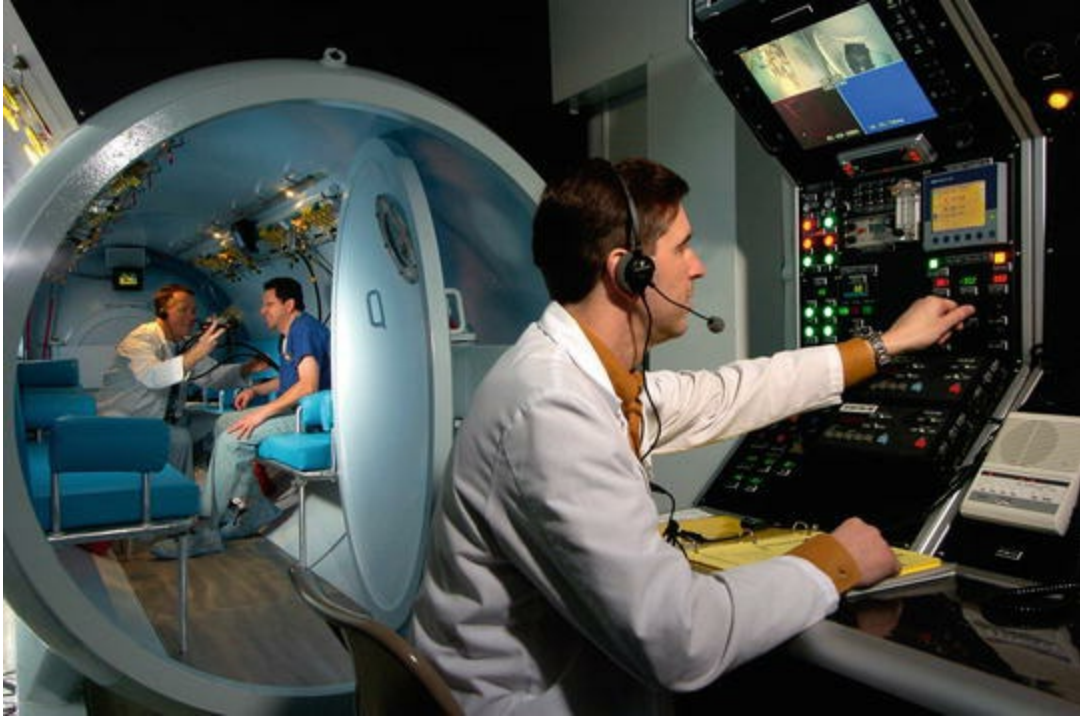
Fig. 7.8 Mobile hyperbaric system interior . An OxyHeal 4000 dual lock, 6 ATA, 12-patient hyperbaric chamber inside a 52' over-the-road trailer, installed adjoining the Emergency Room at Advocate/Lutheran General Hospital in Park Ridge, Illinois, USA. Photo courtesy of OxyHeal Health Group, La Jolla, CA 92038, USA
