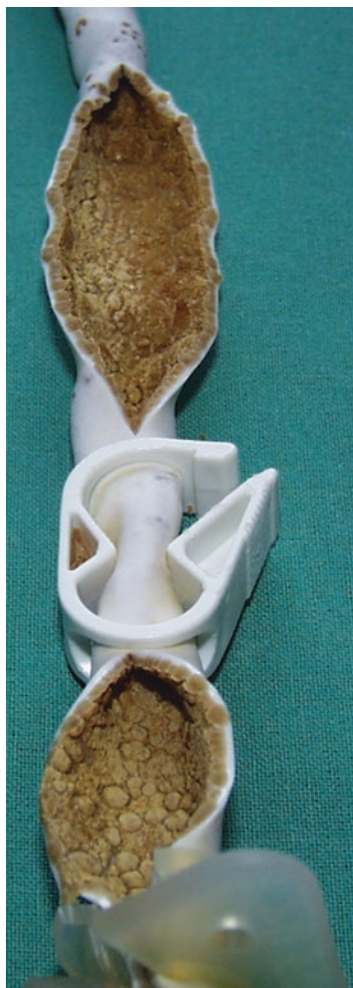
■ Fig. 7.19 Tube obstructed through food residues
