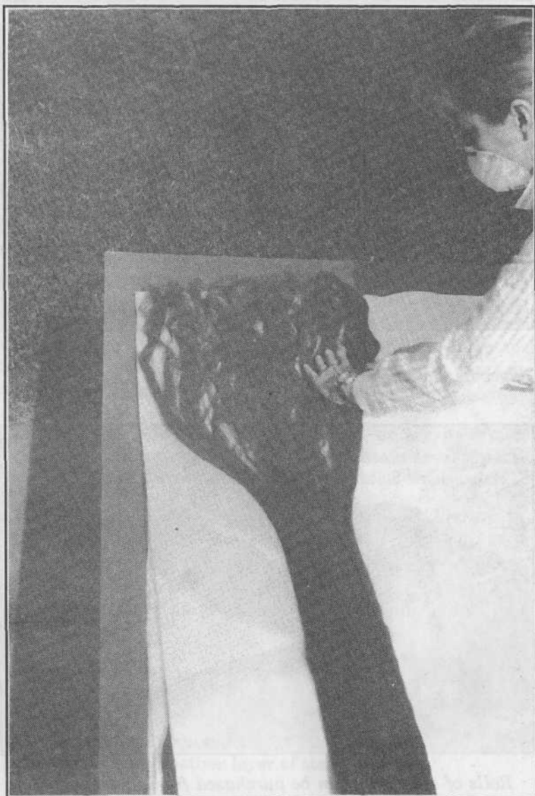
Particle masks should be worn during construction to avoid breathing fine steel dust.
