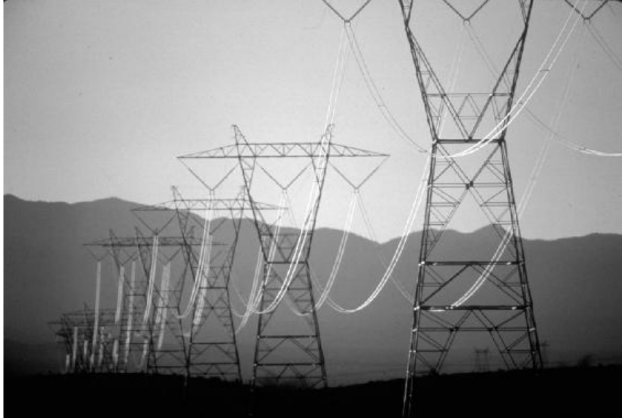
Power lines from Hoover Dam carry electricity to the Los Angeles area. This photo by Charles O'Rear is part of the National Archives digital collection.
