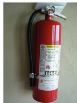
▲ Figure 20.3.4 A fire extinguisher
