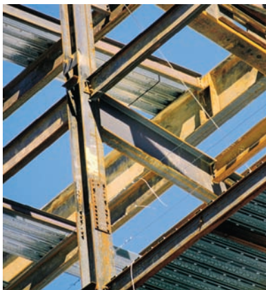
Figure 1.4 As a result of chemical change, bright steel girders become rusty when exposed to moist air.
