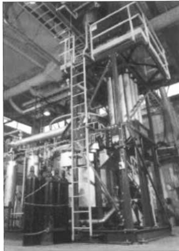
Figure 10.26 Dynamotive 15 t/d fluid bed pilot plant.
