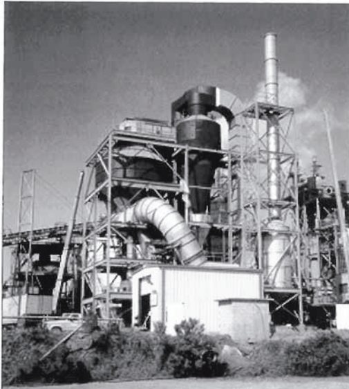
Figure 10.7 SEI Fluid bed gasifier in Florida supplying raw gas for drying.
