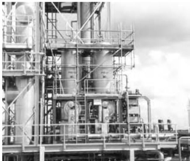
Fig. 25 A pervaporation plant for methanol removal. (View this art in color at www.dekker.com .)
