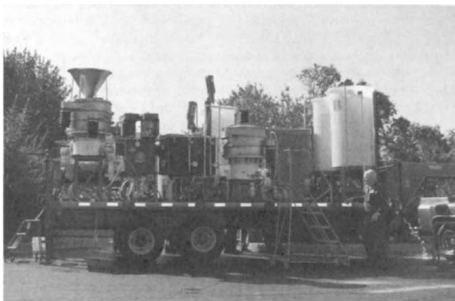
Fig. 6. Portable soil-washing machine shown here at a highway maintenance site used for removal of lead particles from the residue created when bridges and other metal structures are sand-blasted to remove old lead-containing paint. There are numerous applications for such portable plants. (Westinghouse Electric Corporation)
