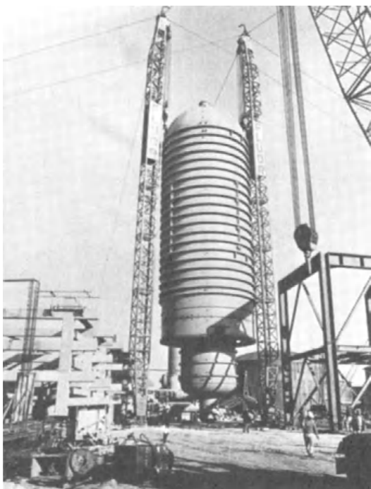
Fig. 3. Erection of 9.5-meter (31-foot) diameter, 263-ton vacuum tower at a petroleum refinery in Kuwait. ( The Fluor Corp )
