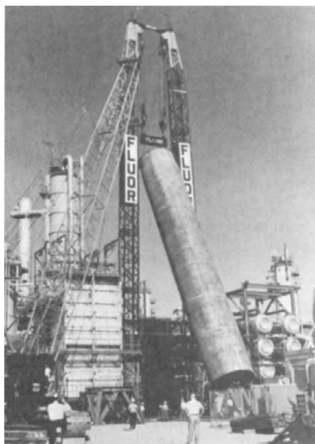
Fig. 4. Erection of a 675-ton hydrocracking reactor at Shauaiba, Kuwait, refinery, the world's first all-hydrogen refinery. ( The Fluor Corp )
