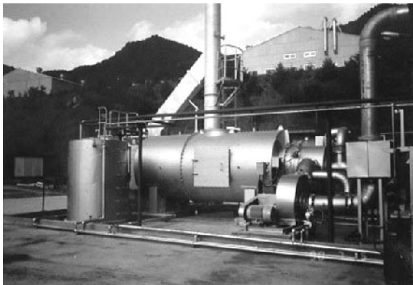
Figure 22.2.13. Energy recovery unit.
