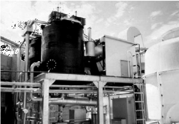
Figure 22.2.10. ACF solvent recovery unit.
