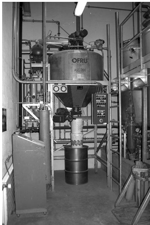
Figure 22.3.4. ASC-200 distillation plant in the explosion-proof room.
