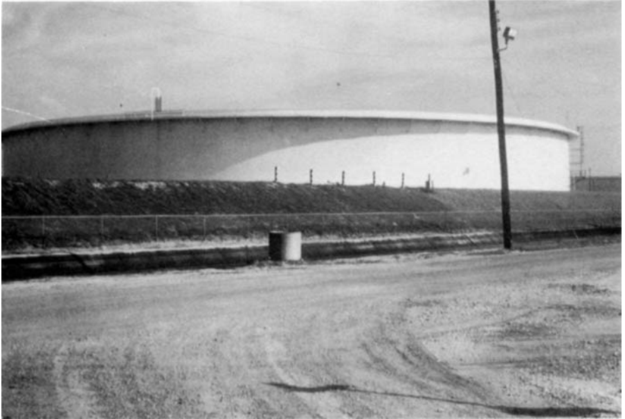
Figure 7.14 Storage tanks for crude oil can be huge. These handle 750,000 barrels, about the size of one oil tanker and perhaps two days supply for the oil refinery. A floating, expandable top enables minimal pressure variation with temperature. (Courtesy of BP Amoco, Texas City, TX)
