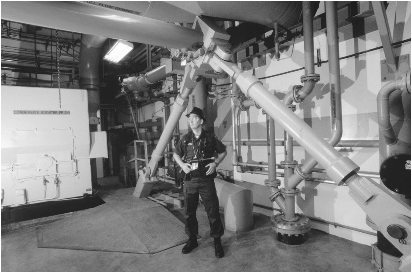
The seismic braces seen here in the Diablo Canyon Nuclear Power Plant reduce the risks associated with an area prone to earthquakes. (Corbis Corporation)
