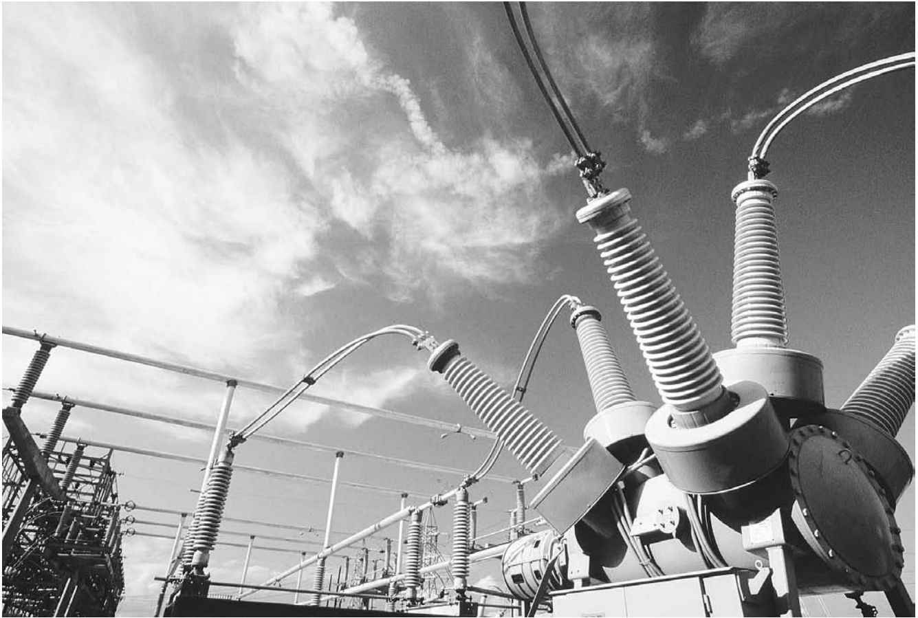
Power transformer station in South Carolina. (Corbis-Bettmann)
