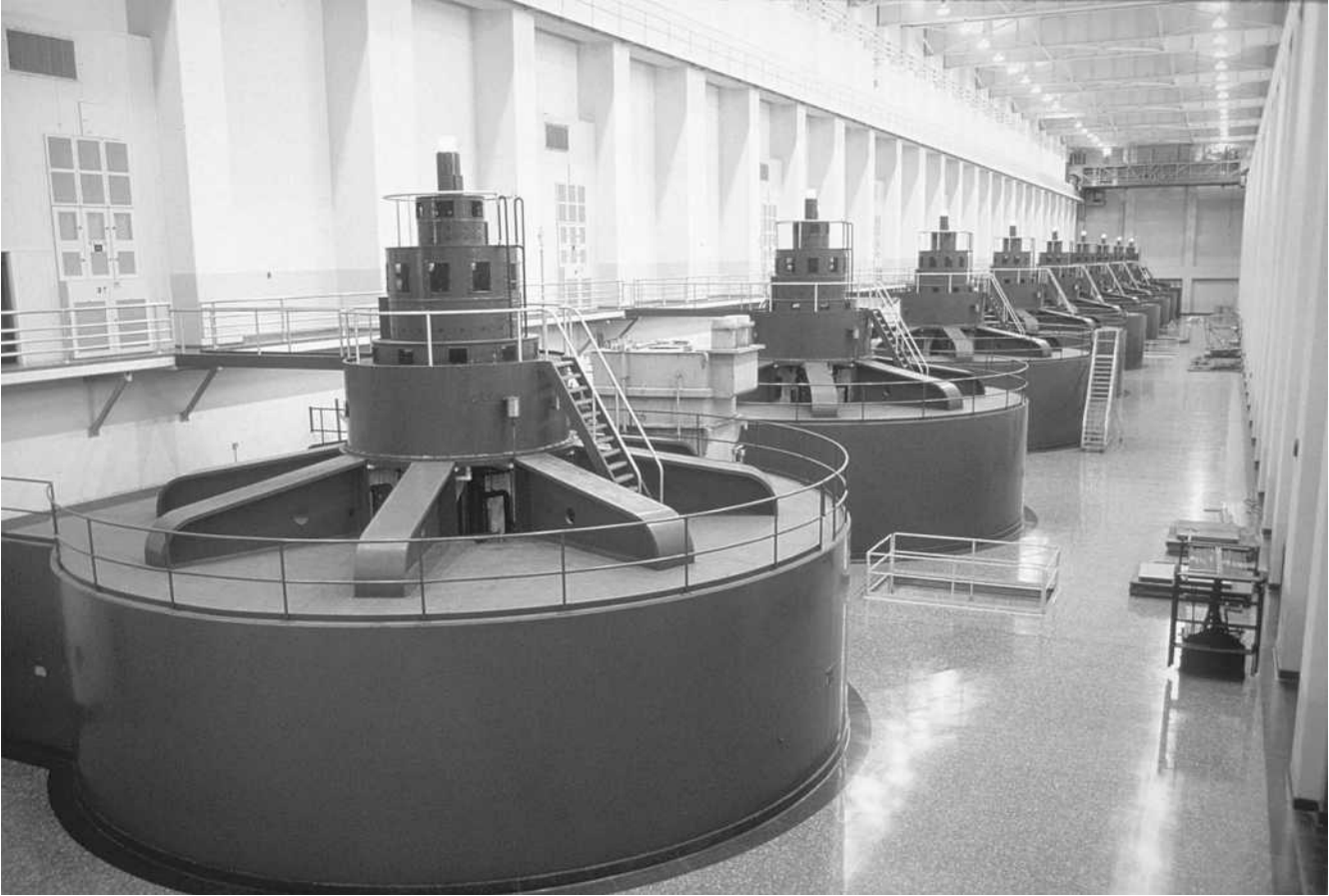
Interior of electrical power plant. (JLM Visuals)
