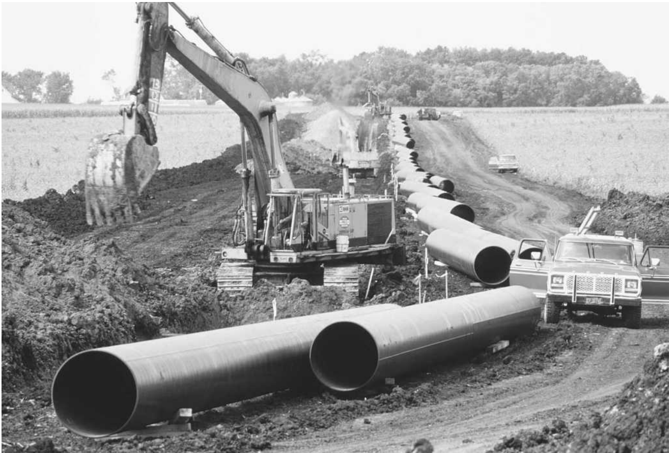
A crane moves soil next to sections of 42-inch pipes to be used for a gas pipeline. (Corbis-Bettmann)
