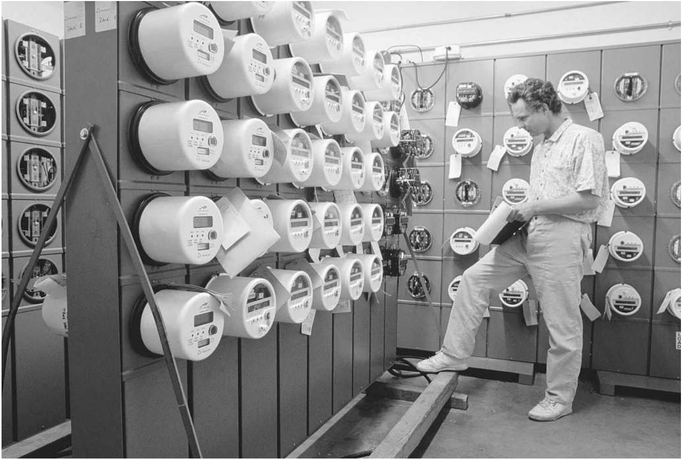
A Southern California Edison employee logs test results at the company's electric meter site. (Corbis-Bettmann)
