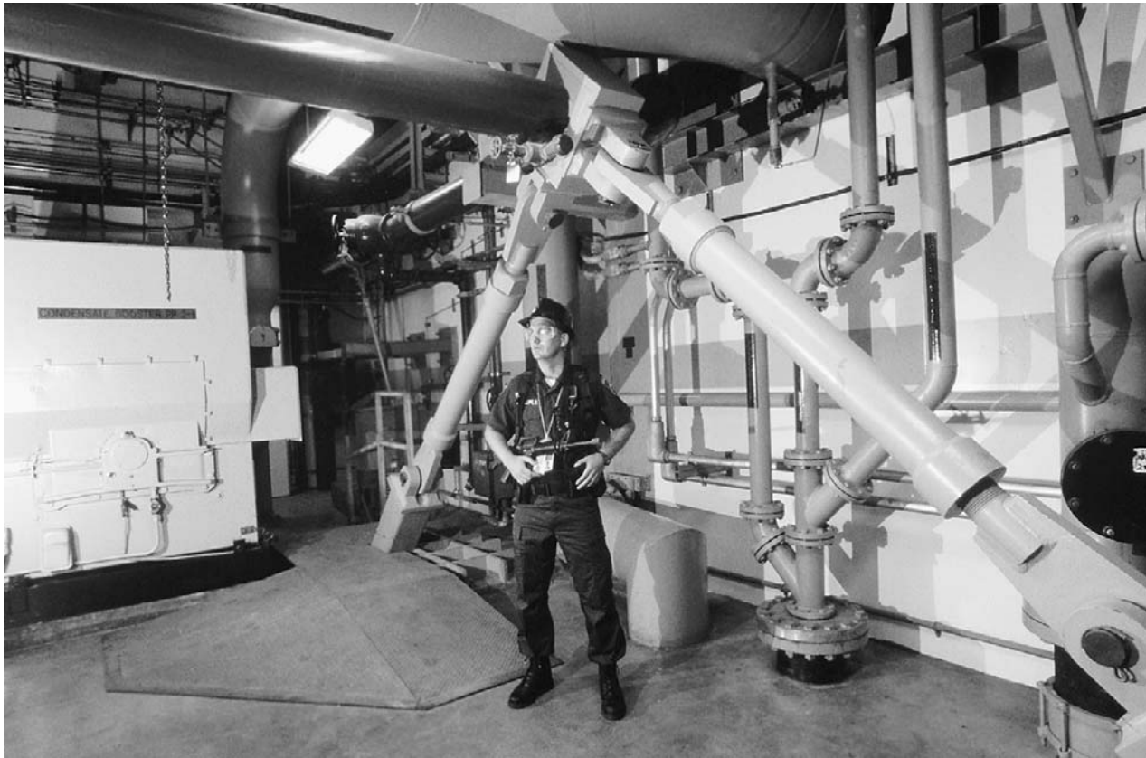
A security officer stands next to a seismic brace inside the Diablo Canyon Nuclear Power Plant. Braces like these are representative of the technological advances in earthquake engineering. (© Roger Ressmeyer/Corbis.)
