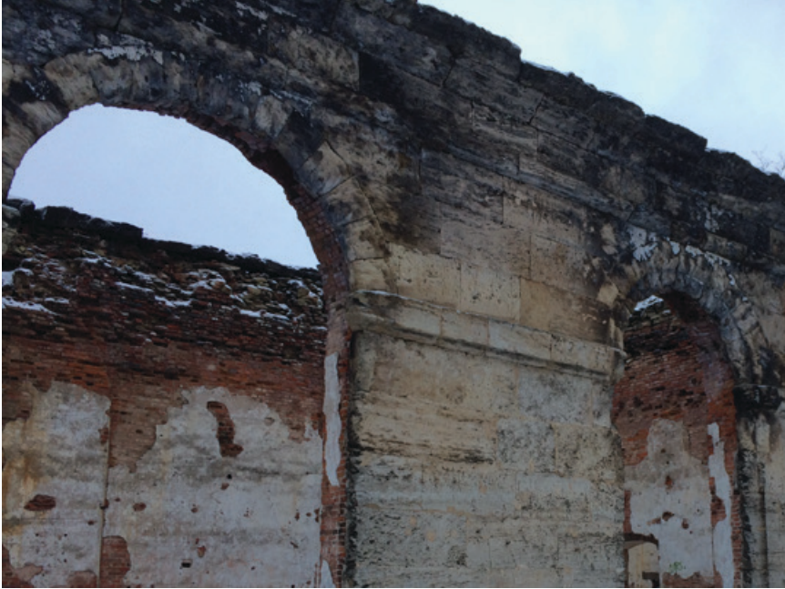
Figure 2.1 The ruin of the Forest Greenhouse ( lesnaia oranzhereia ) on the grounds of the Gatchina Palace Estate Museum, showing the layers of materials that went into its construction: a facing of “Pudost’ stone,” brick interior, and a layer of plaster coating the inside of the walls. Photo credit: © Alison K. Smith.
