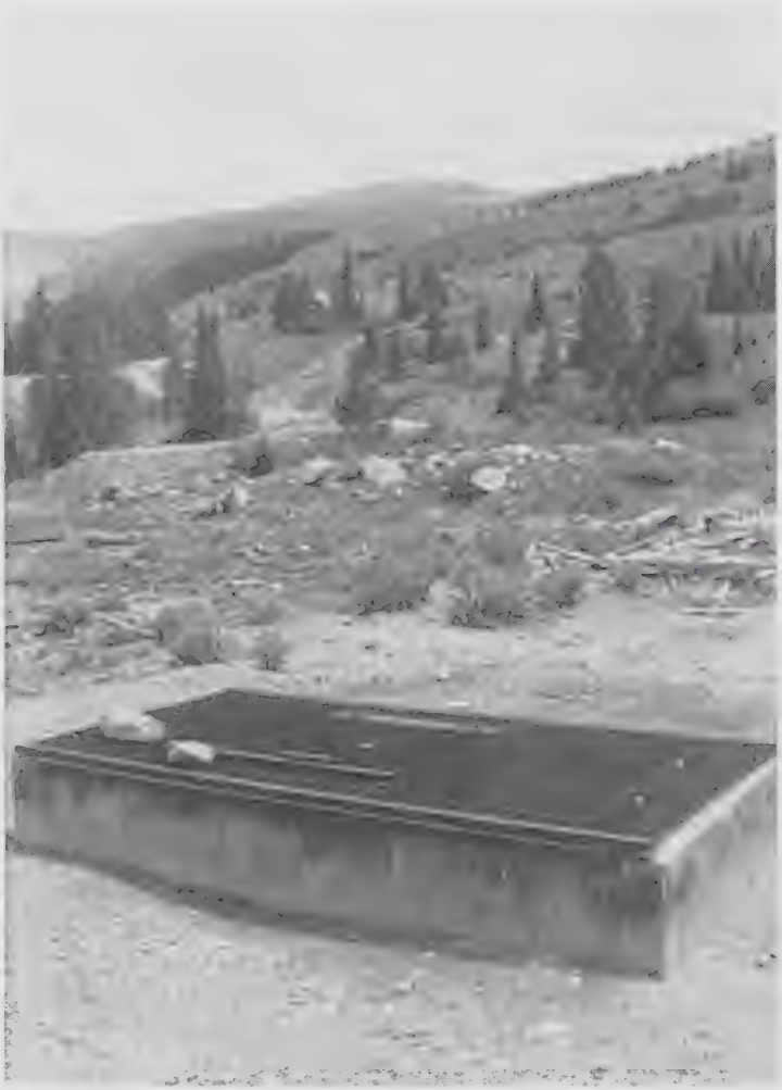
The recently sealed shaft of a hundred-year-old Colorado mine. Three thousand such sites have been made safe by the Colorado Mined Land Reclamation Board.
