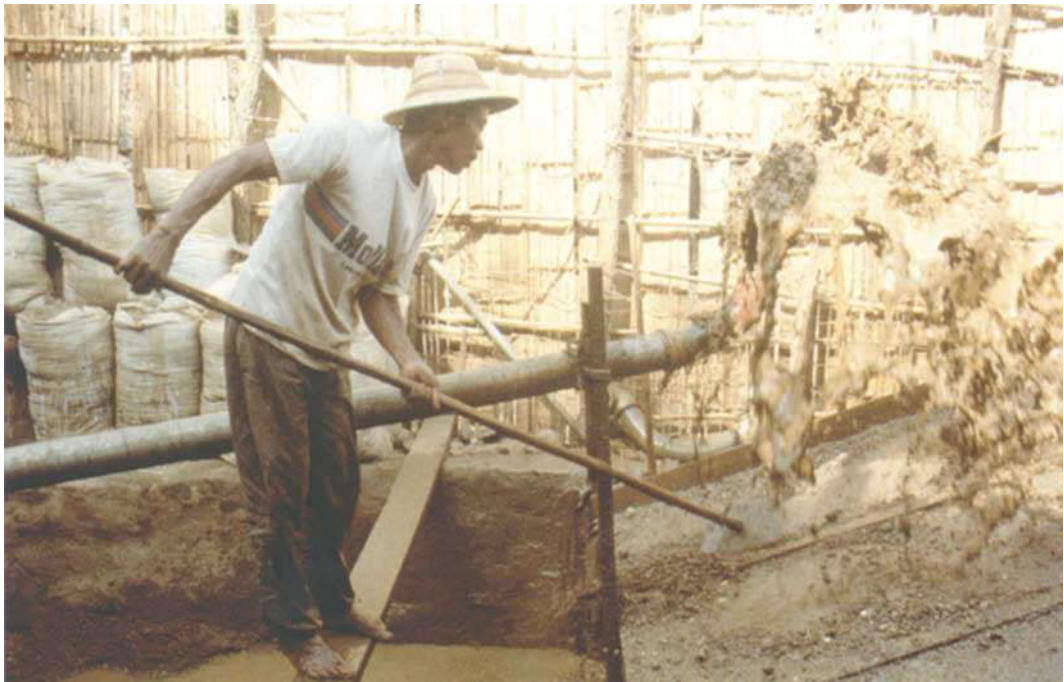
Fig. 11. Gem-laden gravels from the Than Ta Yar mine are pumped to this on-site processing plant where they shower out of a pipe and on to an inclined trough. Photo by R.C. Kammerling
