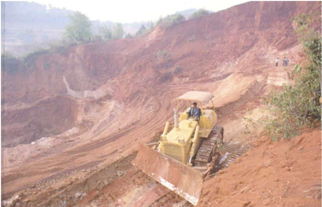
Fig. 10. Removing reddish-brown overburden (from 12-24m thick) to reach the gem gravels at Shwe Pyi Aye. Photo by R.E. Kane
