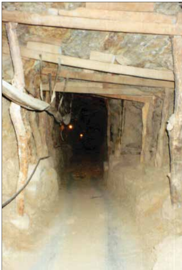
Figure 9: The tunnels at the Scorpion mine have been properly outfitted for a safe and efficient mining operation, with timbering, ventilation, electricity, a concrete floor and a water line, as shown here in the No. 2 decline. Photo by B. Bridges, 2008.
