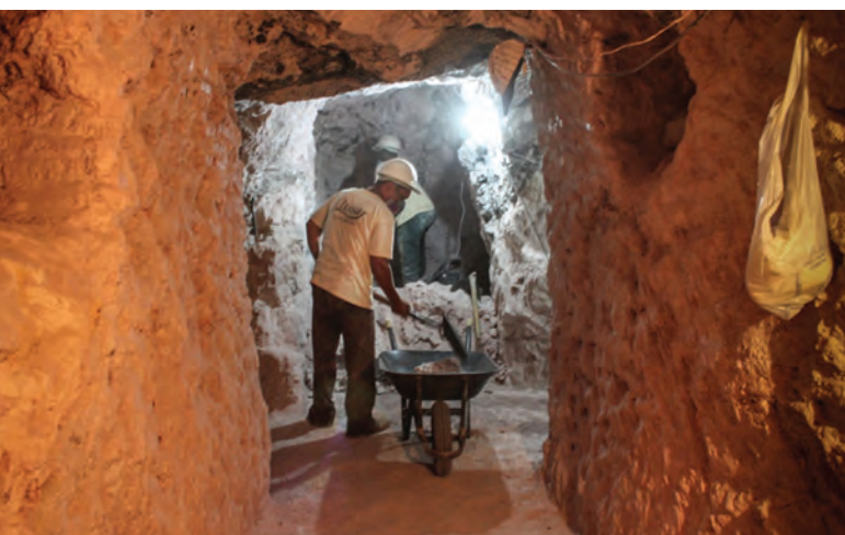
Figure 1: In Bahia State (Brazil), gem-quality rutilated quartz is extracted from tunnels such as this one at the Pyramid mine, owned by Brian Cook. Photo © Brian Cook.
