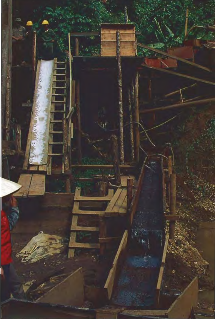
Figure 3. From the pit shown in figure 2, the gem-bearing gravels were pumped to this large sluicing system that, at the time (November 1992), was about 30 m away. The heavy-mineral concentrate collected here, at the end of the system, was then taken to the mine headquarters. Photo by Robert C. Kammerling.
