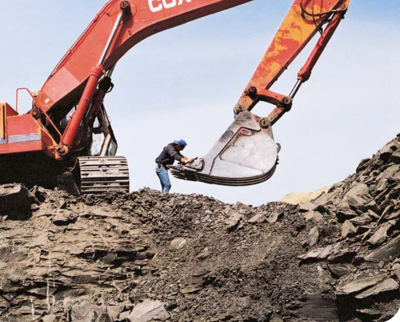
Figure 9. As the backhoe removes the Bearpaw shale at the Oxbow mine, a "spotter" searches the bucket for disk-shaped concretions. Note how friable the shale is. Photo courtesy of Korite International.
