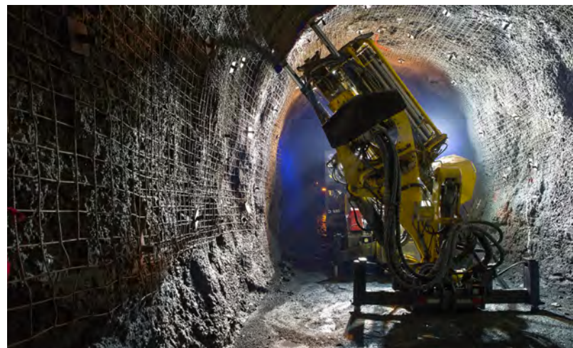
Figure 15. When a tunnel is excavated, this machine is used to install a metal safety screen to prevent debris from falling from the walls or ceiling. Photo courtesy of Diavik Diamond Mine.
