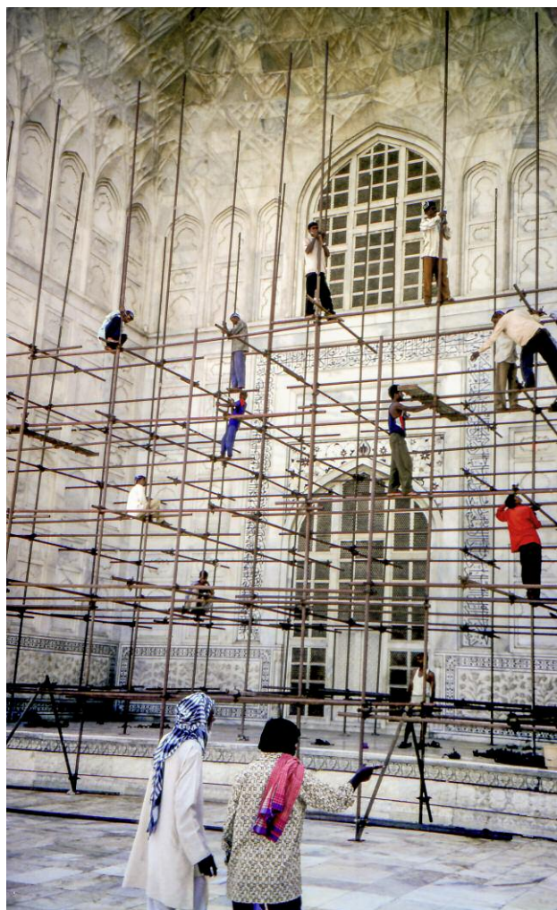
Figure 23. Scaffolding was erected for chemical cleaning of the northern pishtaq of the mausoleum in September 2002. Reproduced with permission of Ebba Koch, 2006.
