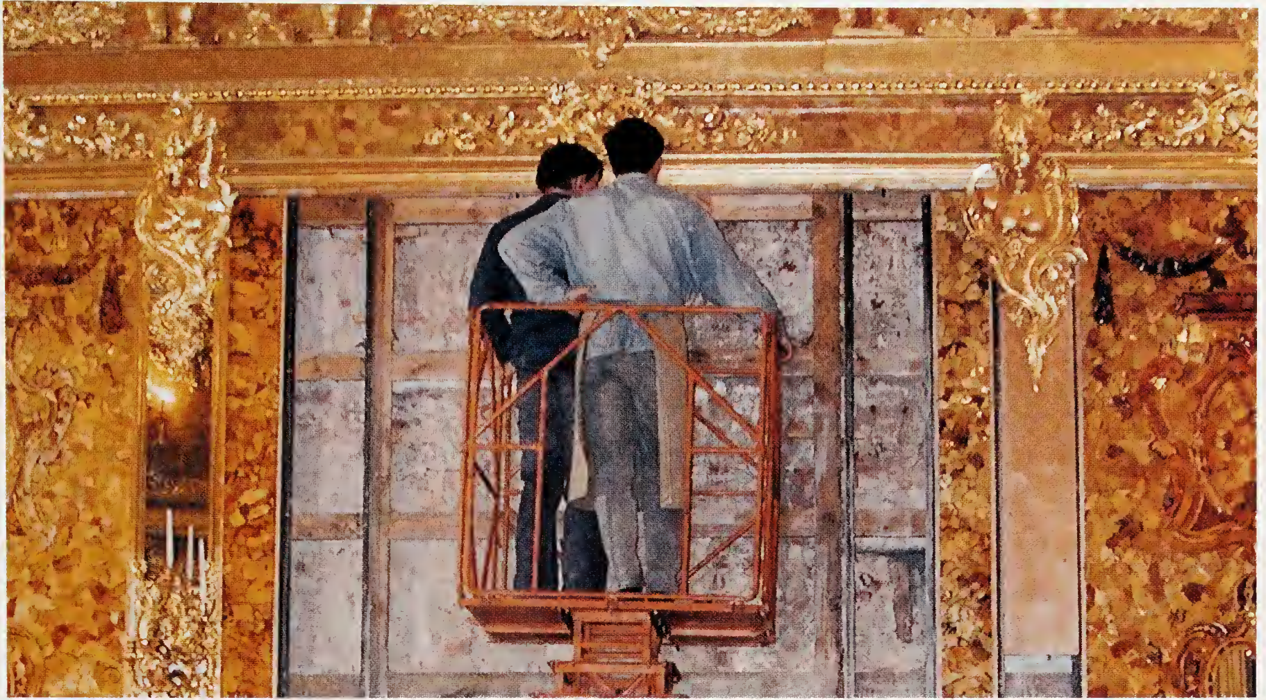
Giving up the search for the lost original: Russian workers during the reconstruction of the north wall of the legendary Amber Room
