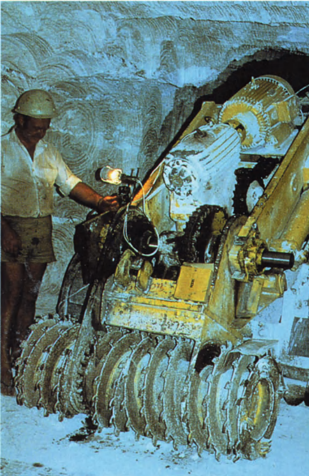
Figure 2-13. Tunneling machine working underground at Coober Pedy, South Australia. Photo courtesy of the Department of Mines and Energy, South Australia.
