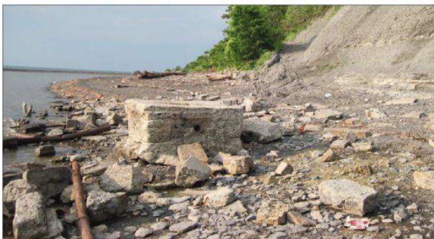
The shoreline along the cliff is littered with blocks of rebar-embedded concrete, as well as limestone.
