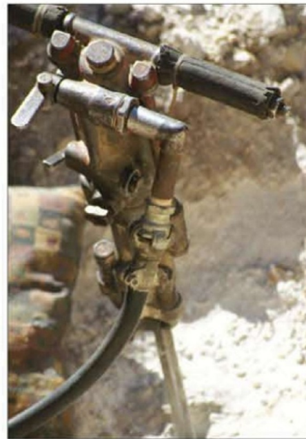
Dennis' jackhammer rests in its borehole while he takes a break from its harsh reverberations.
